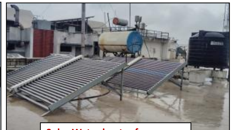
Solar Water heater for Dish washer
